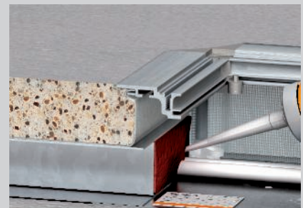
Close the residual joints between cables and blocks with the FBA-SP filler.
