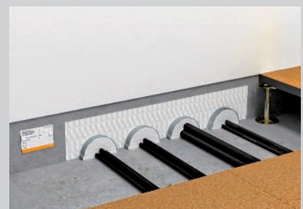
Fully installed half shell in PYROPLATE® Fibre soft insulation.
