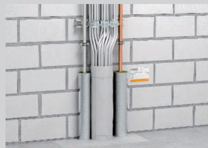
Installation of the fire protection bandage with no distance to the Rockwool Conlit pipe insulation.
