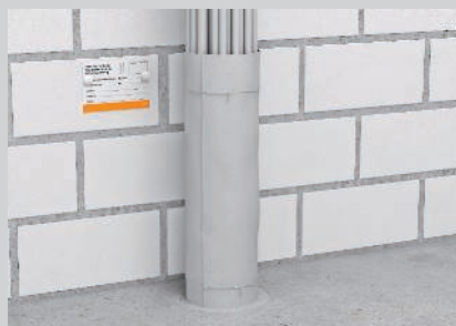
Using mortar, close off the residual insulation opening and mount the identification plate.
