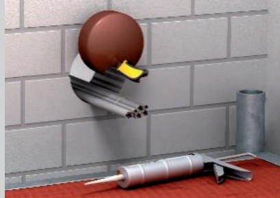
Cutting of the plugs for cable assignment on the edge of the core hole.
